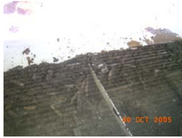
Scale falls off of the condenser tube
