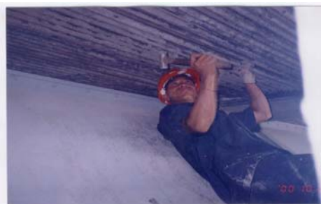
Knocking scale off the system
