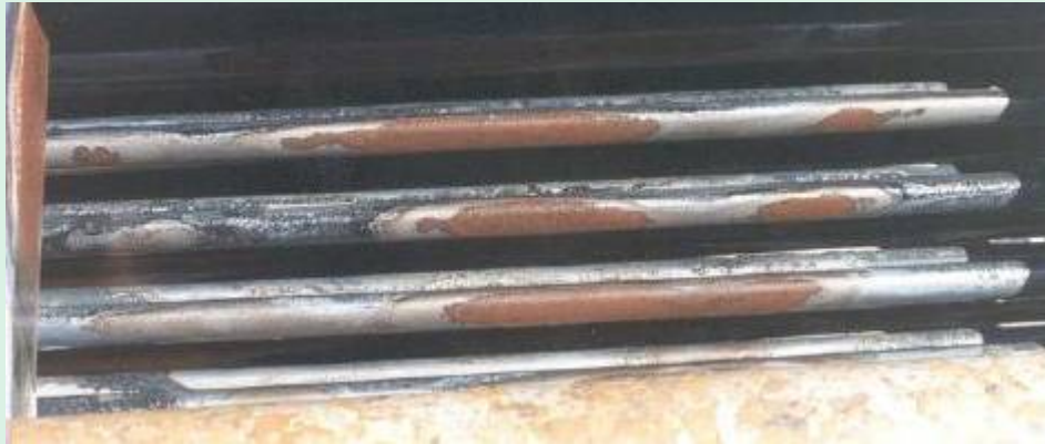
Cooling System Tube Bundles Ruined by Improper Acid Treatments
